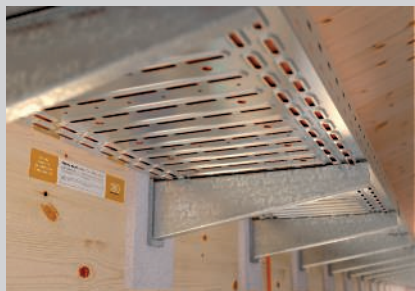
Bracket mounting on the side of the wooden beam with rear fire protection plate.
