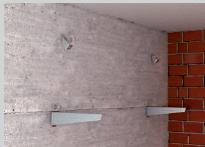
Mounting of the brackets and the sloping connection components on a wall.
