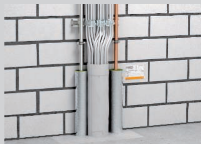
Installation of the fire protection bandage with no distance to the Rockwool Conlit pipe insulation.
