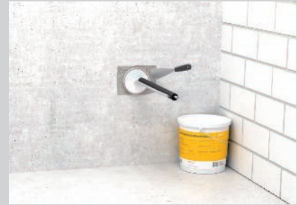
Adjust the foam plugs to installations using a knife and create smoke gas-tight sealing of the sealings using the ASX coating compound.
