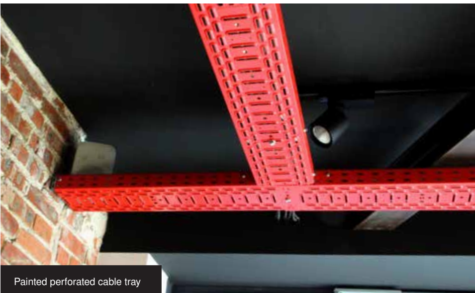
Painted unperforated cable tray Brezel Museum, Erdmannhausen
